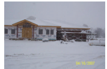
The Town Hall at 93 E Main. This is what the Town Hall looked like 3 years ago today.
